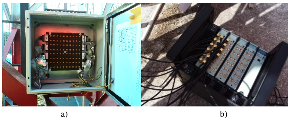
Fig. 3. a) Patching panel; b) data acquisition unit
